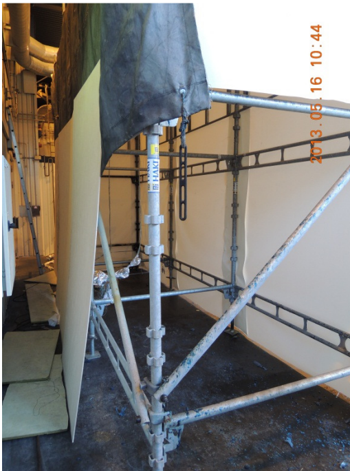
Figure 20 Rear-side of the supporting structure covered with non-combustible fabric and non-combustible board.
