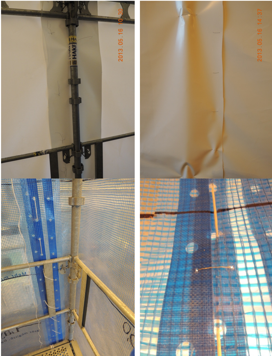
Figure 23 Techniques used to bind the sheets together and to the supporting structure (top left: binding of PVC membrane to supporting structure from the inside | top right: binding of PVC membrane to supporting structure from the outside | bottom left: binding of weather protection membrane to supporting structure from the inside | bottom right: binding of weather protection membrane to supporting structure from the outside).
