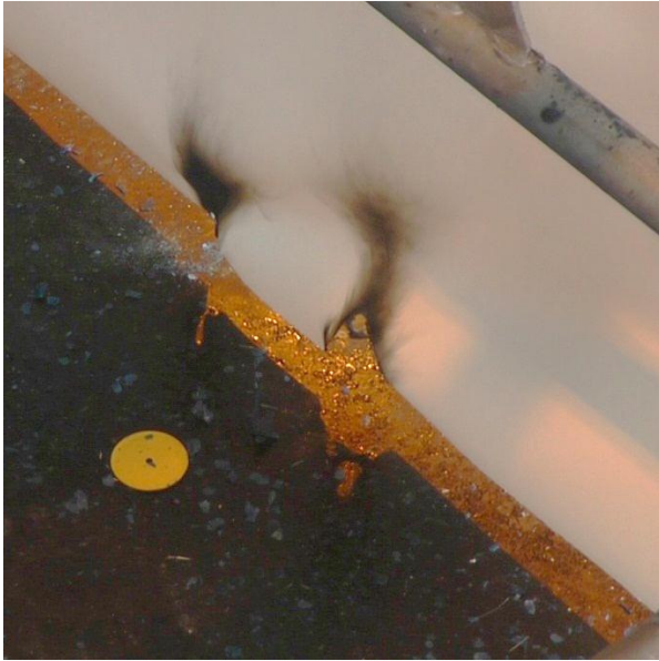
Figure 70 Fire damage after edge exposure from the inside (right: 30 s flame exposure; left: 15 s flame exposure).
