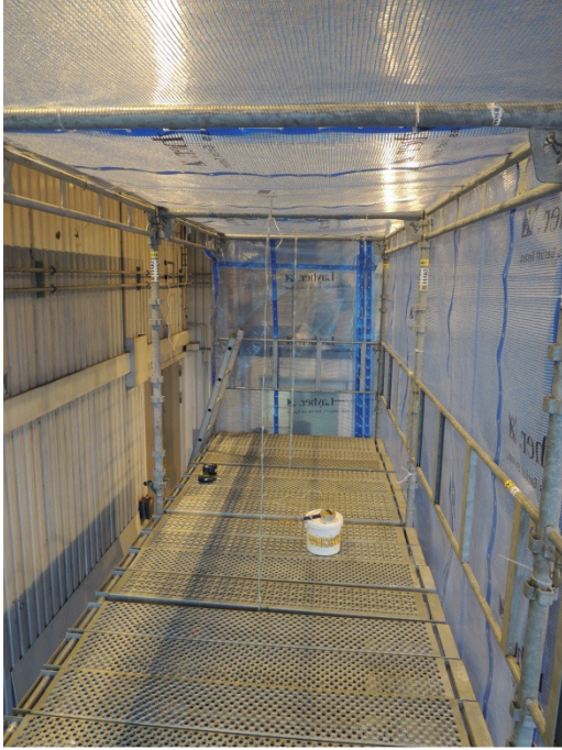
Figure 15 Inserted floor made of perforated steel separates the first from the second floor.
