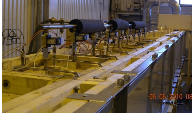
Figure 5 A photo of the water supply system for the automatic water sprinklers
